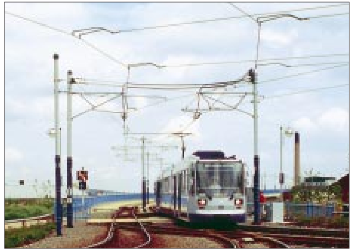
Fig. 4: Fibre ropes used to support tramway cables in the absence of insulators
